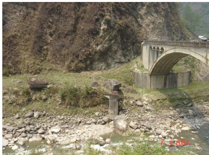
Remnant of a bridge destroyed by the 1981 Zhanzanbo GLOF alongside the bridge constructed after the GLOF
